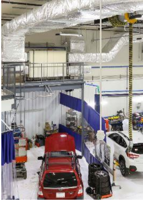
For its anniversary, a car dealership in the Canadian town of Alberta treated itself to a new showroom complete with a workshop, all built to the Passive House standard. © Garret Scott
